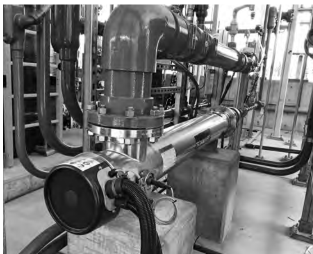
A view of the Regional Recycled Water Program demonstration facility.
